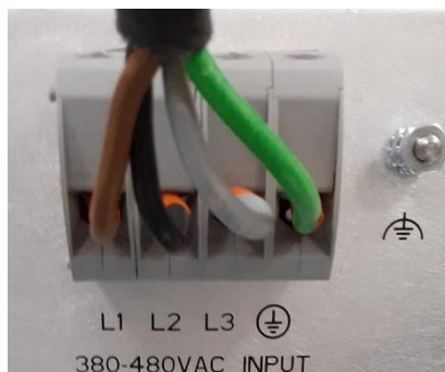
Figure 56 - Three-phase terminal strip
